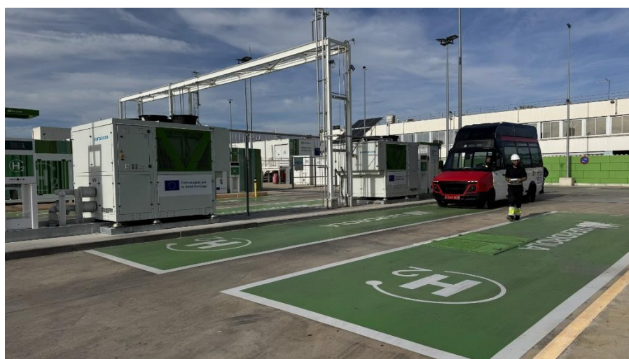
Figure 14. Hydrogen refuelling station in the Barcelona Free Zone. Source: J.R. Morante
